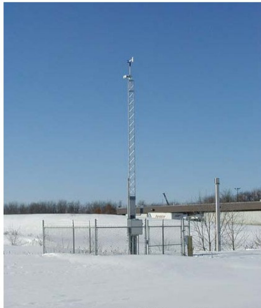
Typical Canadian RWIS installation
